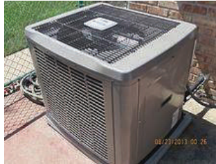
Figure 3.1.1.1 Condenser unit for crucial aircon for a regular residence
